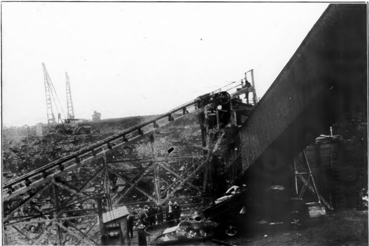
Truck Discharging Into Primary Crusher. Conveyor at Left Elevates Stone to Primary Grizzly. Building at Right is Housing For Conveyor to Screens Over Bins
